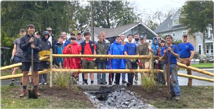
Boy Scout Troop 815 and one of their completed erosion projects in Section 1.
